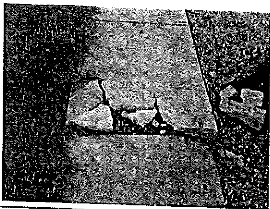
Grade F – Not present, broken, and/or impassable.
