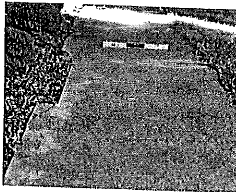
Grade C – Major/Multiple Deficiencies: For instance, the sidewalk shown here is too narrow and has bad cross slope.
